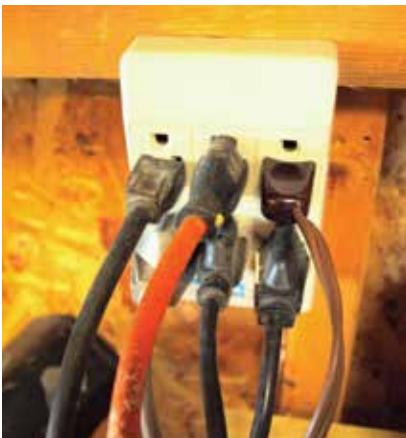
Avoid overloading outlets with adapters and too many appliance plugs.
